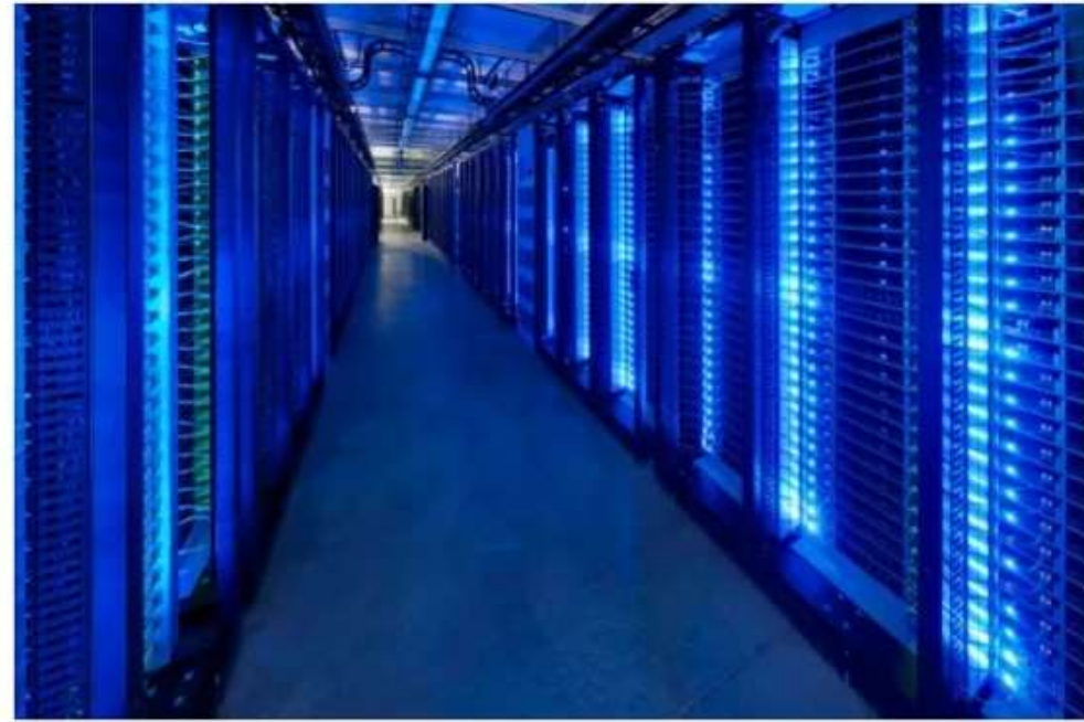
Source: Interior of one of Google's Data Center, www.google.com/about/datacenters/
